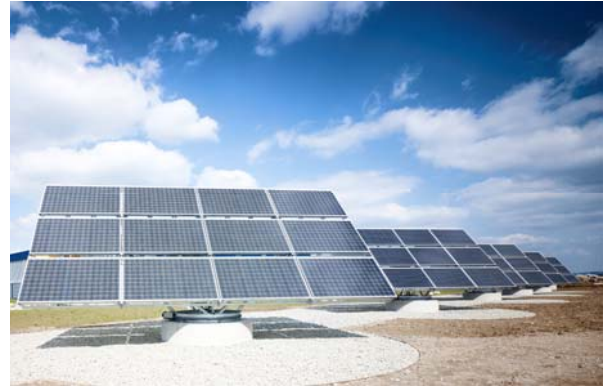
Figure 9 – Photovoltaic installation (ERSOL)
